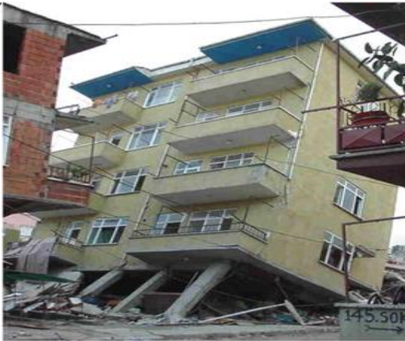
(a) Open story failure
