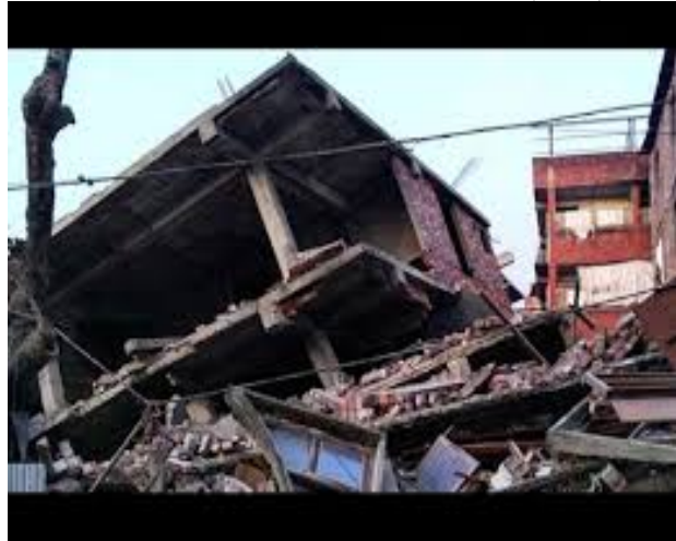
(b) Out of plane failure
